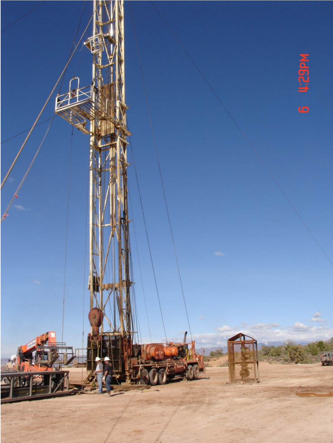
Monument work-over rig on Paradox Basin #3 (Note Paradox Basin #1 wellhead in cage)
